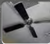
Two (2) Ceiling Fans (Bedroom and Living Area)
